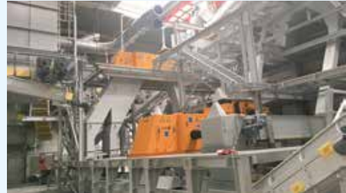
New recycling plant Diksmuide operational
